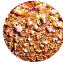
Varnish on reservoir ceiling (Stalactites)
